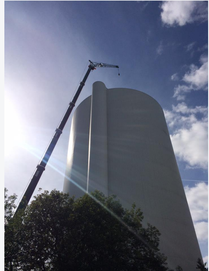
SSV hot water storage tank
